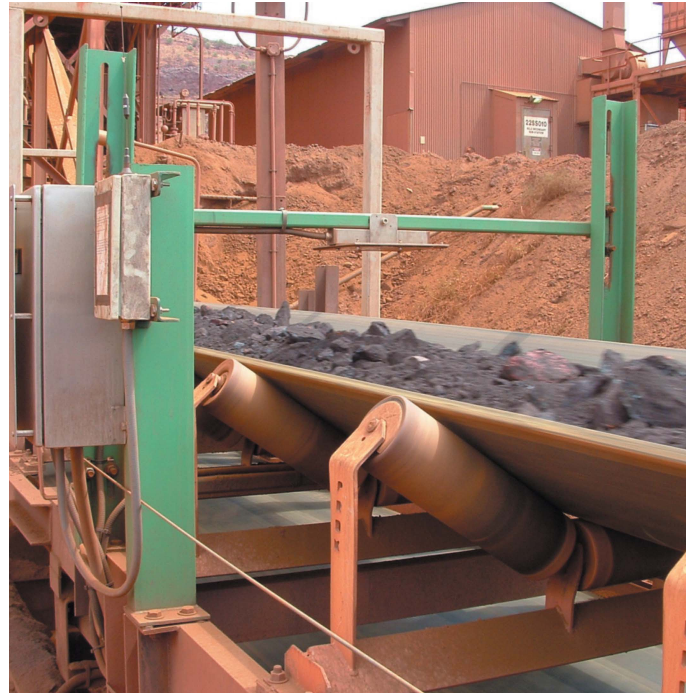
LFM Pilbara Moisture Analyser operating at Whaleback Mine.
